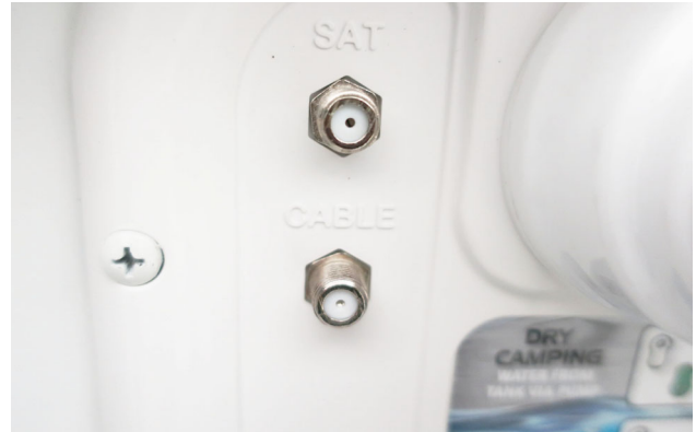
Satellite Dish and Cable TV Connections (Located on the Water Center Panel) -Typical View
