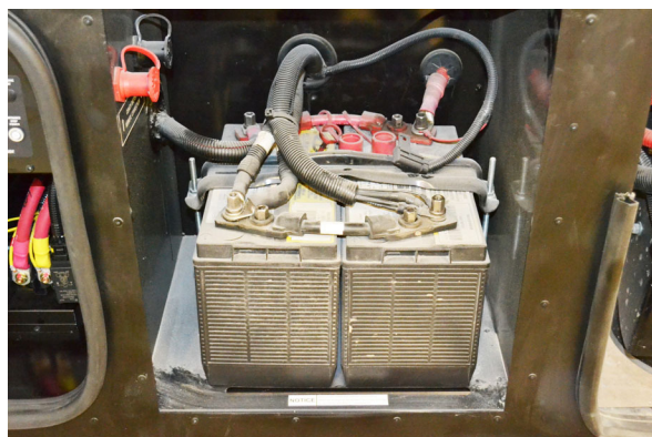
Chassis Batteries -Typical View
