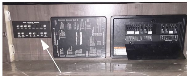
House Circuit Breakers -Typical View
